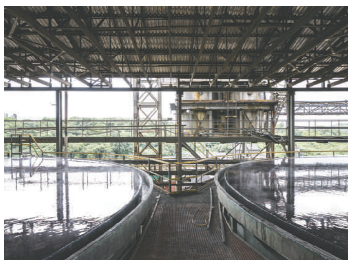
Manganese ore from the Kalahari is dissolved in huge vats of sulfate solution at the MMC refinery in Mbombela.
